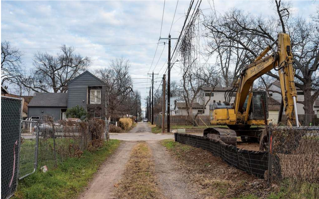
A recent flattened lot next to two new builds. Photograph by Marie Ketring
